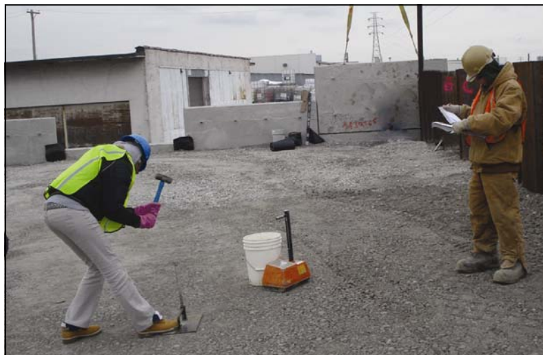
L-R: Senior Jessica Flanigan and Josh Cambridge employee with the City of St. Louis-Civil Engineering Department at the Jefferson Avenue bridge replacement.
